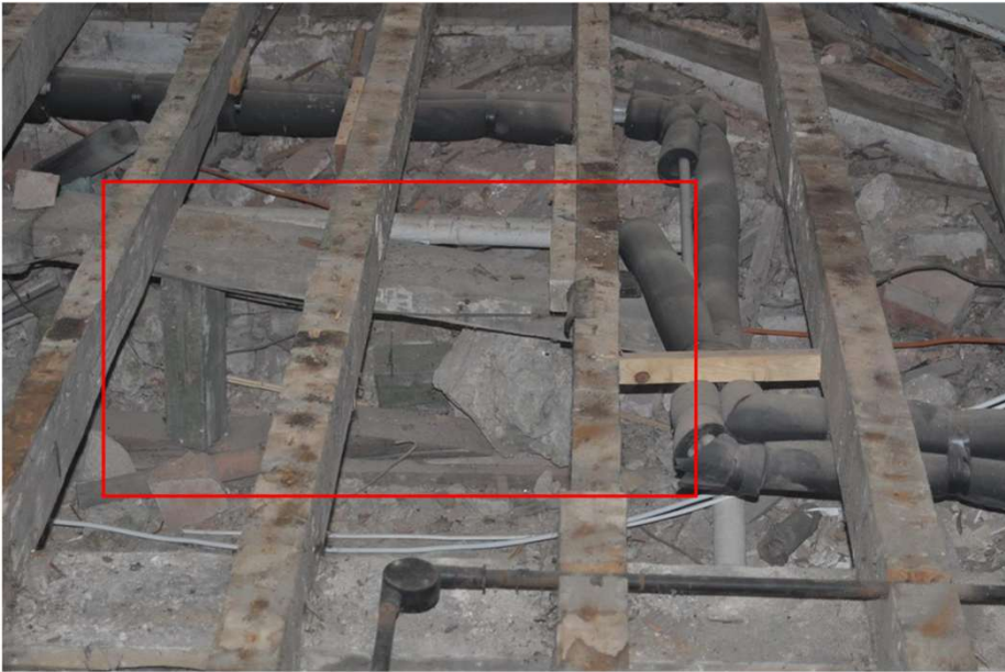
Figure 12. Displaced and unsupported headplate.
